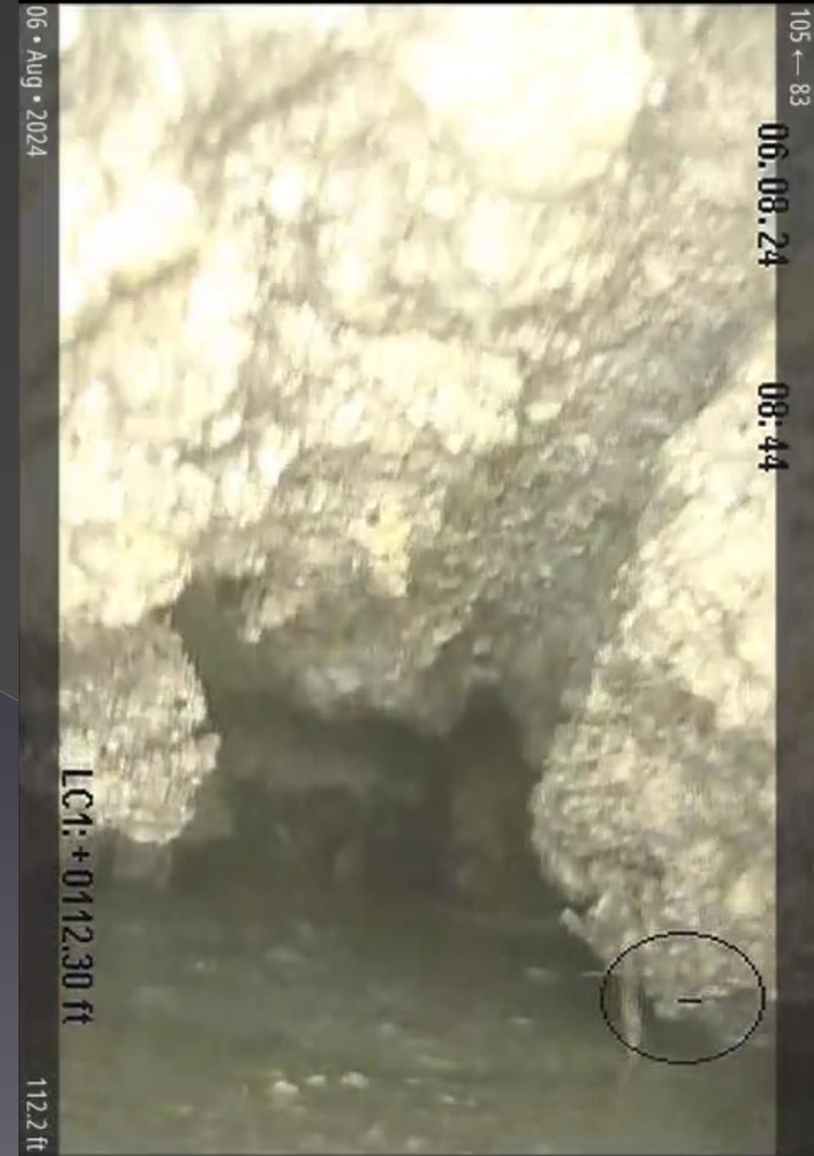
FOG Buildup on Sewer
