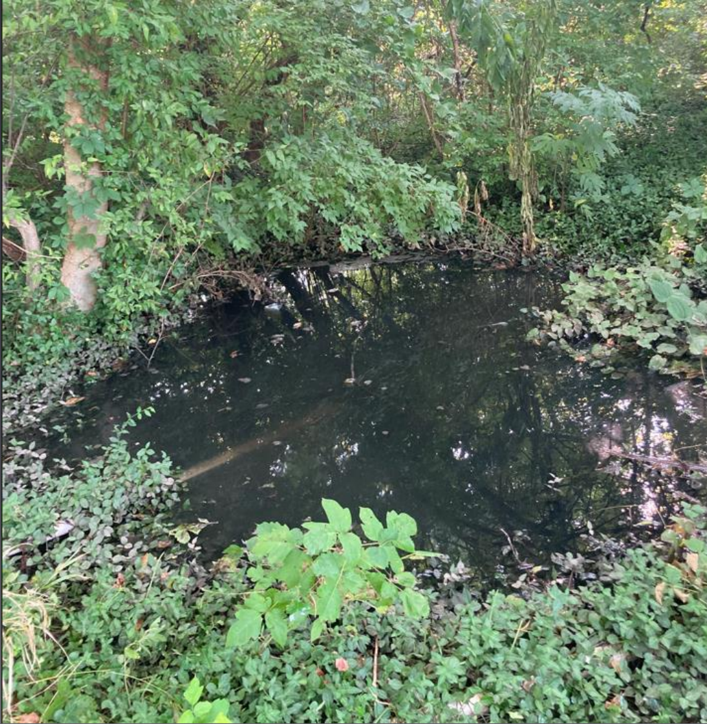
Submerged Sewer Manhole & Bypass Pipe
